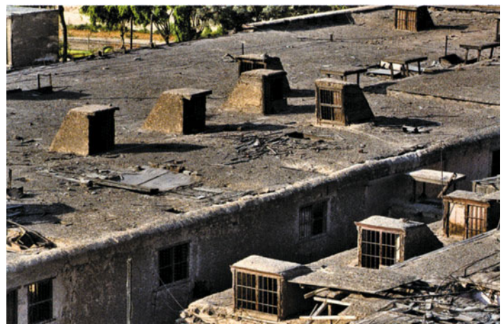
TEATINA-QUINCHA SHELTER, PISCO, PERU, ALEXIA LEÓN. VIEW OF TEATINAS ON THE ROOF OF AN OLD WAREHOUSE.
